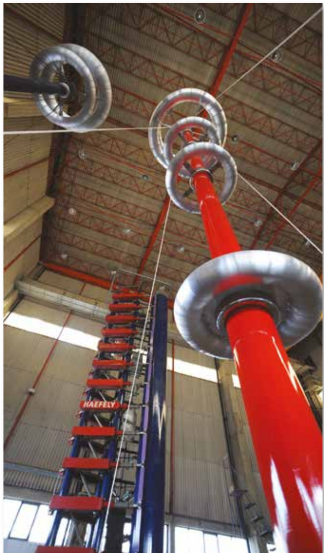
Lightning impulse generator voltage divider.
